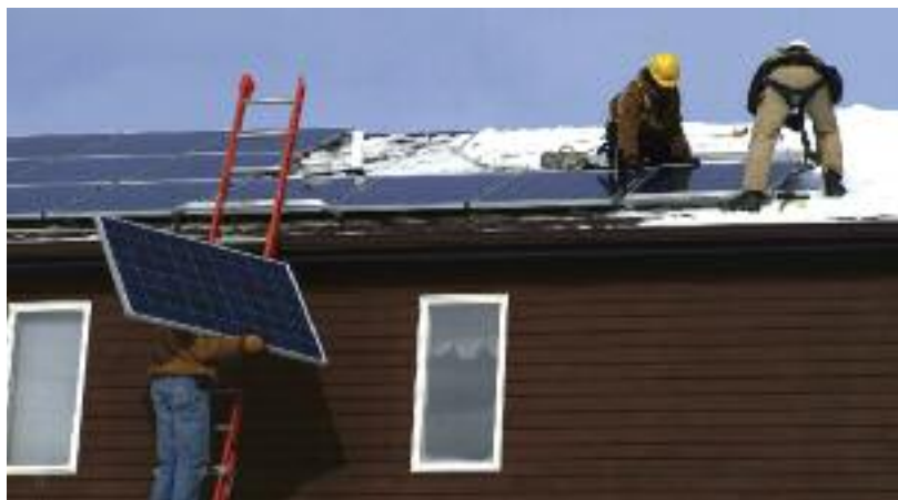
Solar panels installed at a Solar Williston home
