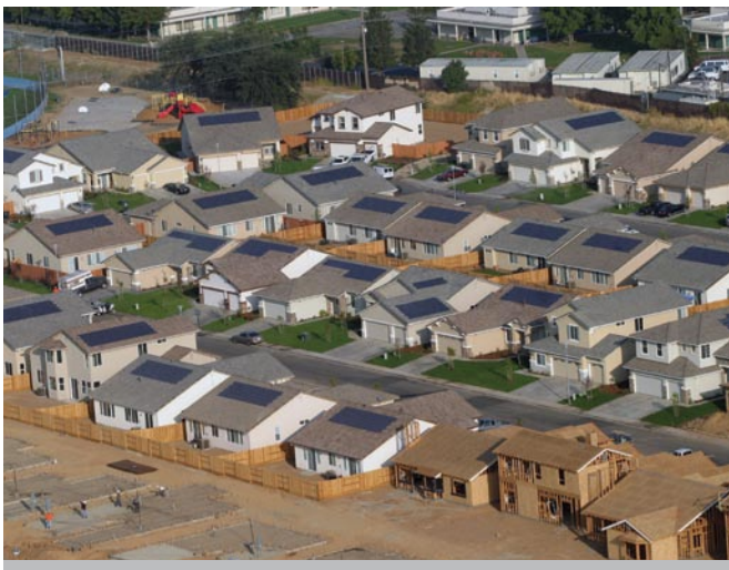
Zero energy homes, like those under construction in this Sacramento subdivision, couple energy-efficient design with small-scale renewable energy generation to dramatically reduce consumption of fossil fuels. (Credit: Sacramento Municipal Utility District)
