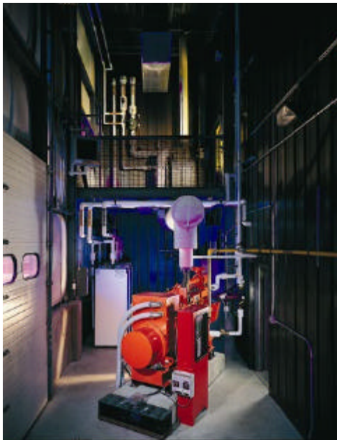
Small scale, customer sited, Combined Heat and Power applications, like this one recently installed at Green Mountain Coffee Roasters, provide a number of important benefits to Vermont's economy and energy mix.
